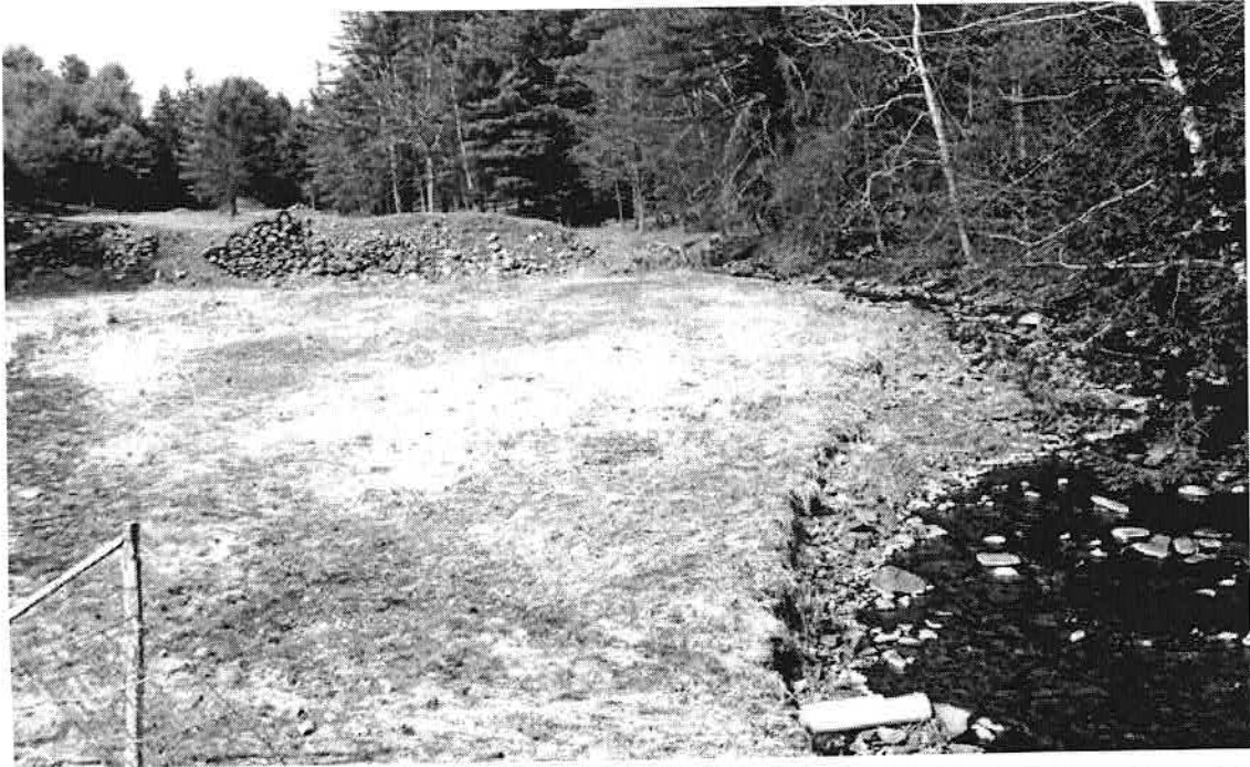
The earthen dam on Drake Hill Rd, near intersection with CR 41 and Sunny Hill Rd; JdBakkerKill on right.
