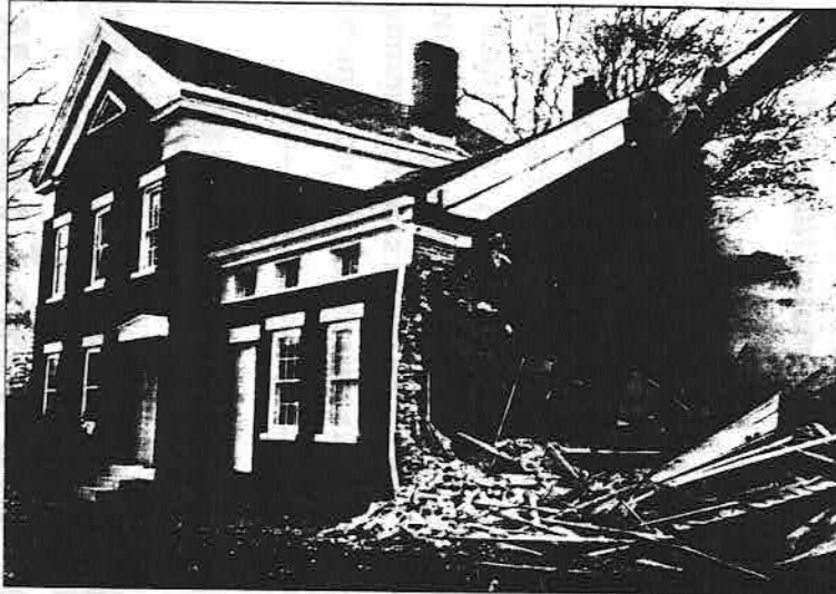
The historic Sherrill House, circa 1845, was razed last Monday afternoon despite efforts to save it.
